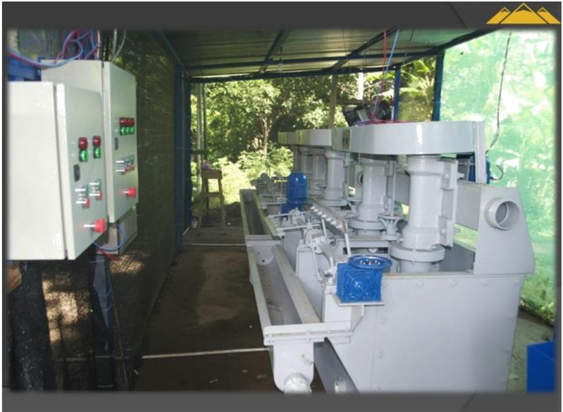
Figure 7 – Processing facility, Oro Roca S.A., Los Juntas
