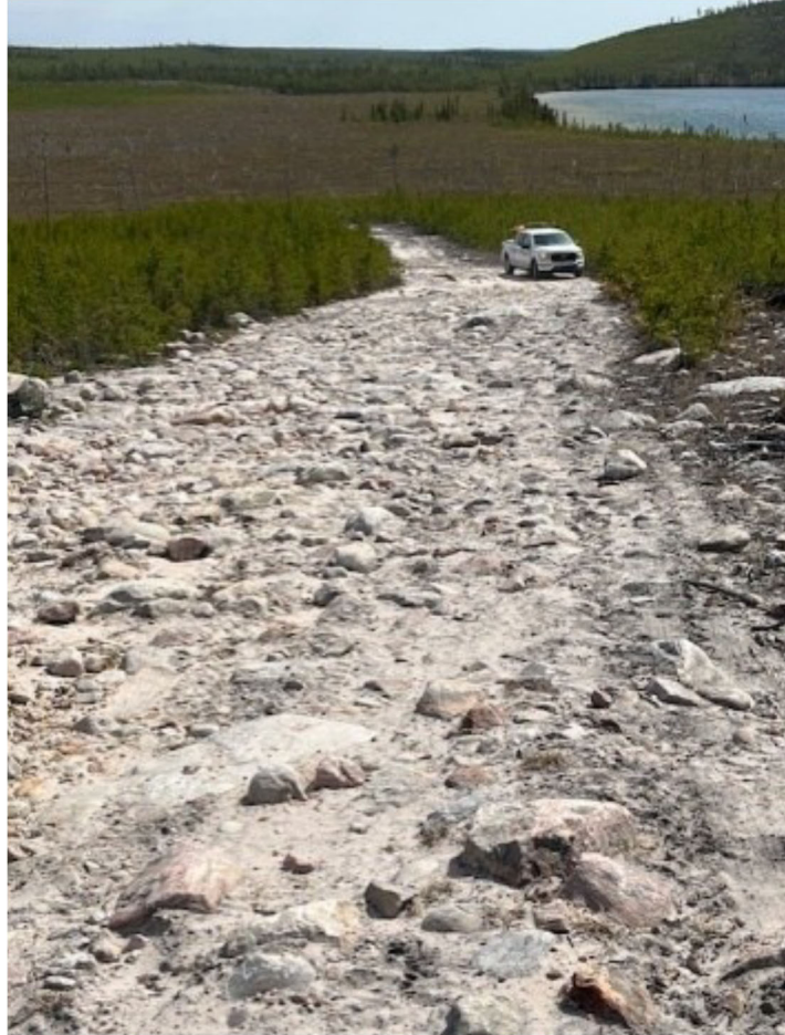
Figure 12-3 Washout on Claim Block MC 00014551
